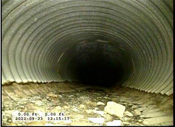
1, 00:00:11, 0.00ft Catch Basin / CB5
