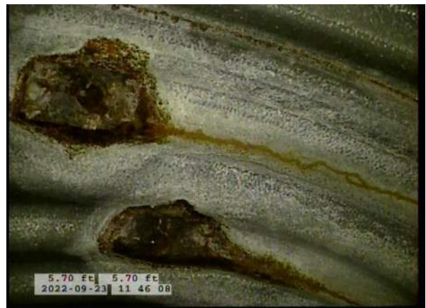
8, 00:01:52, 5.70ft Infiltration Stain from 1 o'clock to 3 o'clock
