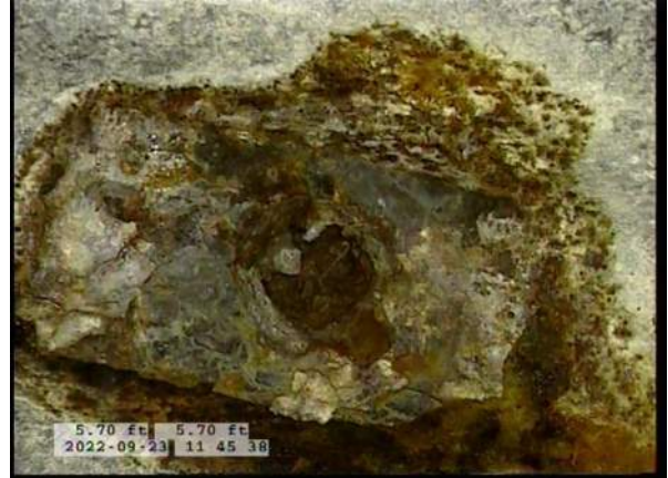
6, 00:01:29, 5.70ft Surface Damage Missing Wall from 1 o'clock to 2 o'clock / SMALL HOLES
