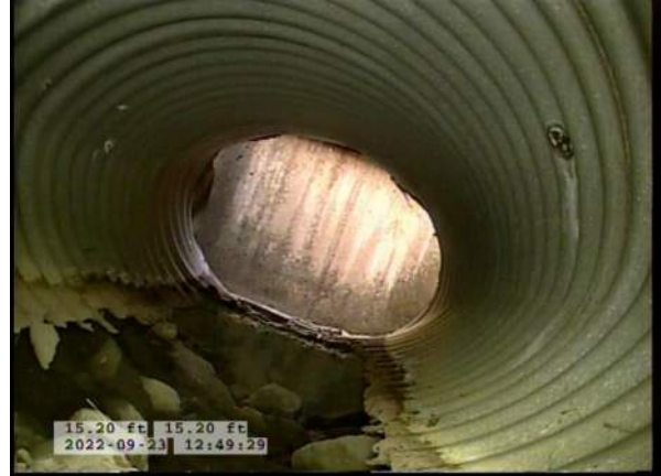
10, 00:02:27, 15.20ft Surface Damage Missing Wall from 5 o'clock to 7 o'clock, within 8 inch, Finish / BOTTOM OF PIPE HAS BEGUN RUSTING AWAY
