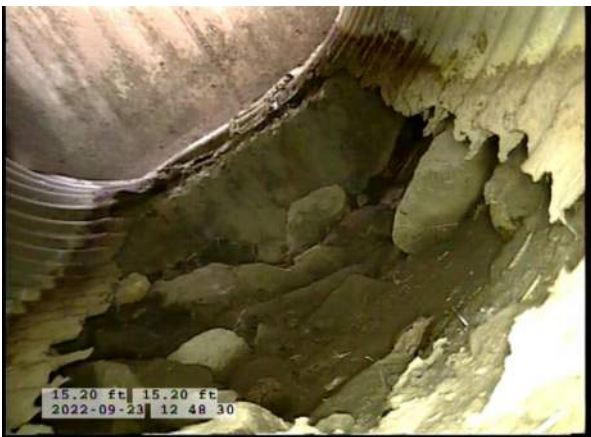
7, 00:01:56, 15.20ft Miscellaneous General Photograph from 5 o'clock to 7 o'clock / BOIIOM OF PIPE COMPLETELY MISSING JUST BEFORE CB4
