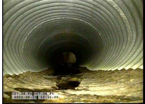
18, 00:14:36, 167.04ft Deposits Settled Fine, 5% of cross sectional area from 6 o'clock to 7 o'clock, within 8 inch, Finish
