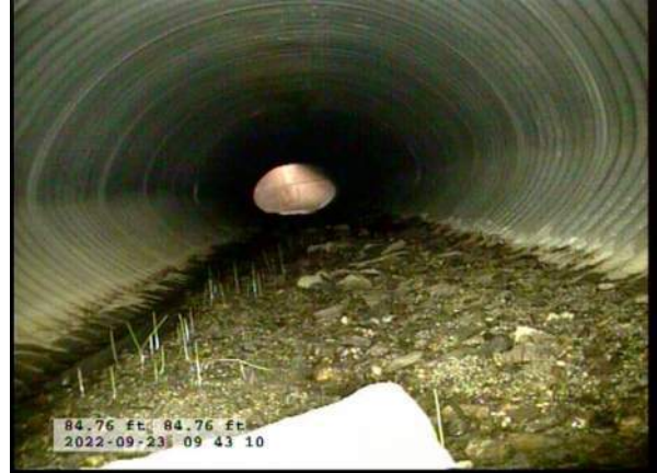
10, 00:04:32, 84.76ft Deposits Settled Gravel, 5% of cross sectional area from 5 o'clock to 7 o'clock, within 8 inch, Start
