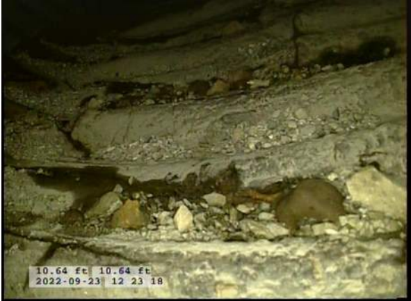
9, 00:02:44, 10.64ft Surface Damage Missing Wall from 5 o'clock to 7 o'clock, within 8 inch, Start / BOTTOM OF PIPE HAS STARTED TO RUST AWAY
