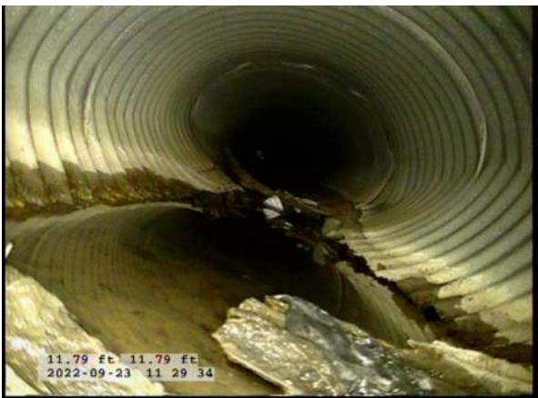
7, 00:02:29, 11.79ft Surface Damage Missing Wall from 5 o'clock to 7 o'clock / BOTTOM OF PIPE HAS RUSTED AWAY
