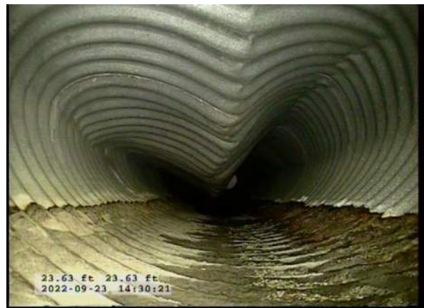
8, 00:01:47, 23.63ft Collapse, 80% of cross sectional area
