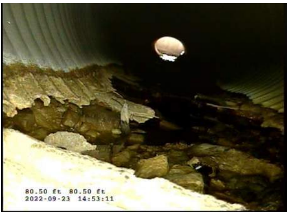
7, 00:04:39, 80.50ft Miscellaneous General Photograph from 5 o'clock to 7 o'clock / BOTTOM OF PIPE COMPLETELY MISSING
