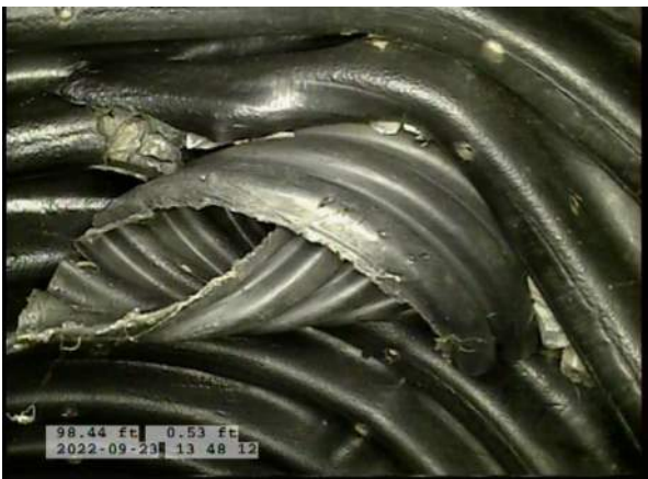
3, 00:05:26, 0.53ft Tap Break-In Defective at 1 o'clock, dia/height: 3inch / CRUSHED END OF PIPE ON LATERAL
