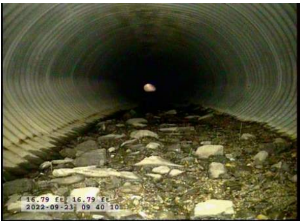
7, 00:02:00, 16.79ft Deposits Settled Gravel, 5% of cross sectional area from 5 o'clock to 7 o'clock, within 8 inch, Start
