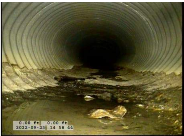
3, 00:00:16, 0.00ft Deposits Attached Encrustation, 5% of cross sectional area from 5 o'clock to 7 o'clock, within 8 inch, Start / RUST
