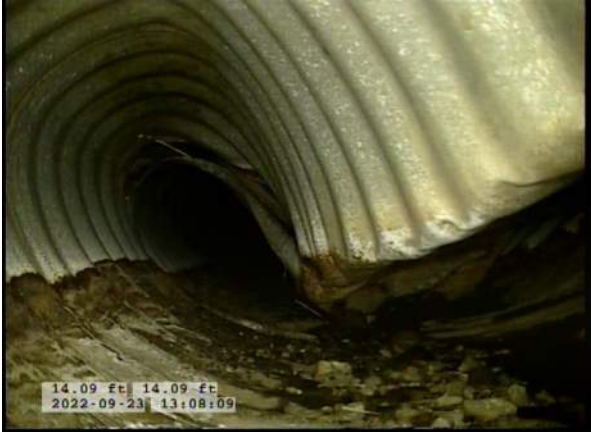
9, 00:03:08, 14.09ft Deposits Attached Encrustation, 5% of cross sectional area from 5 o'clock to 7 o'clock, within 8 inch, Finish / RUST
