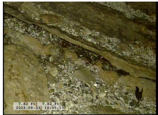
4, 00:01:06, 7.82ft Surface Damage Missing Wall from 5 o'clock to 7 o'clock / BOTTOM OF PIPE STARTING TO RUST AWAY
