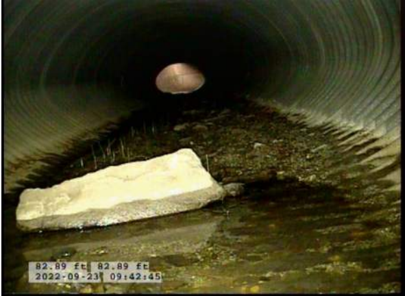
9, 00:04:22, 82.89ft Obstruction Rocks, 5% of cross sectional area from 6 o'clock to 7 o'clock
