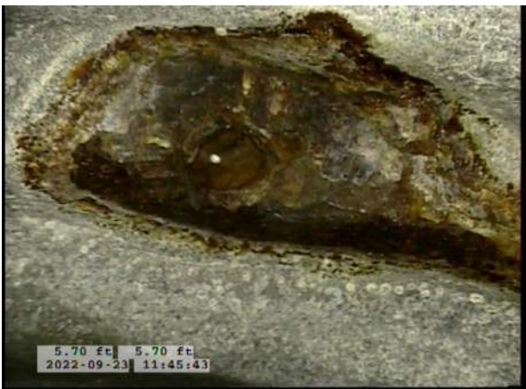
7, 00:01:29, 5.70ft Surface Damage Missing Wall from 1 o'clock to 2 o'clock / SMALL HOLES
