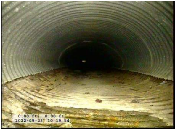
1, 00:00:11, 0.00ft Catch Basin / CB9
