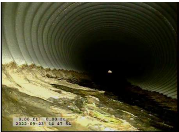
3, 00:00:23, 0.00ft Deposits Attached Encrustation, 5% of cross sectional area from 5 o'clock to 7 o'clock, within 8 inch, Start / RUST
