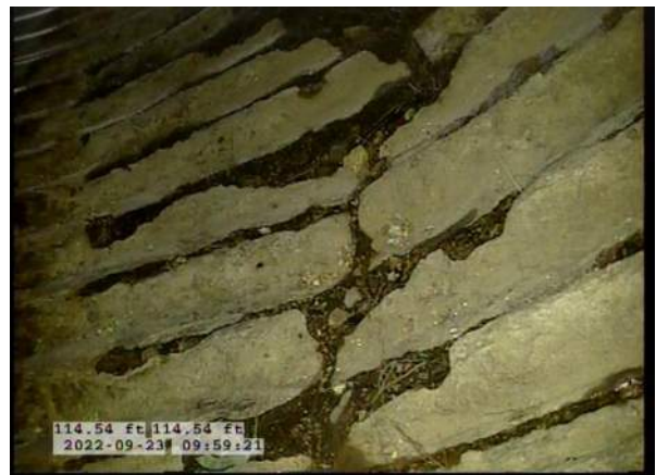
12, 00:06:50, 114.54ft Miscellaneous General Photograph from 5 o'clock to 7 o'clock / BOTTOM OF PIPE RUSTING AWAY
