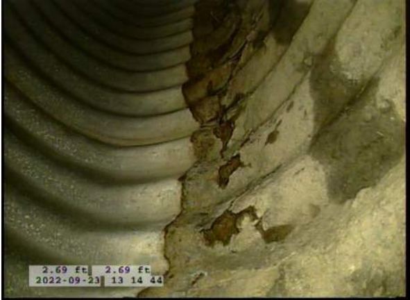
5, 00:00:44, 2.69ft Surface Damage Missing Wall from 5 o'clock to 7 o'clock, within 8 inch, Start / BOTTOM OF PIPE HAS BEGUN RUSTING AWAY
