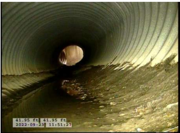
15, 00:06:26, 41.95ft Surface Damage Missing Wall from 4 o'clock to 7 o'clock, within 8 inch, Finish / BOTTOM OF PIPE HAS BEGUN RUSTING AWAY
