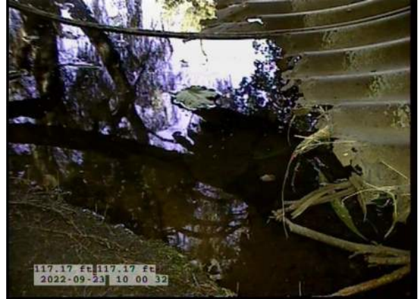
14, 00:07:26, 117.17ft Miscellaneous General Photograph from 5 o'clock to 7 o'clock / BOTTOM OF PIPE COMPLETELY MISSING AT END OF PIPE
