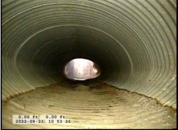
1, 00:00:10, 0.00ft Catch Basin / CB9
