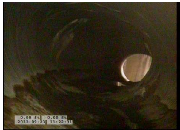
8, 00:01:43, 0.00ft Miscellaneous General Photograph from 12 o'clock to 12 o'clock / ZOOMING CAMERA DOWNPIPE, CB8 VISIBLE
