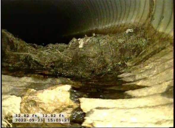
9, 00:01:51, 12.82ft Miscellaneous General Observation / BITTOM OF PIPE COMPLETELY MISSING
