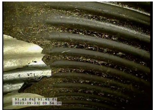
8, 00:03:14, 91.43ft Miscellaneous General Observation / BITUMINOUS COATING ON THIS LENGTH OF THE PIPE
