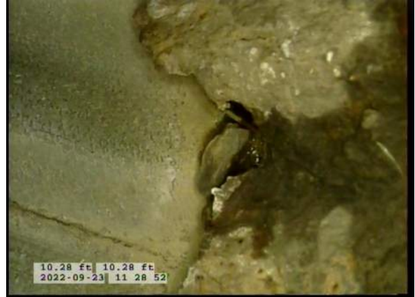
6, 00:01:59, 10.28ft Surface Damage Missing Wall from 7 o'clock to 8 o'clock / SMALL HOLES FORMING
