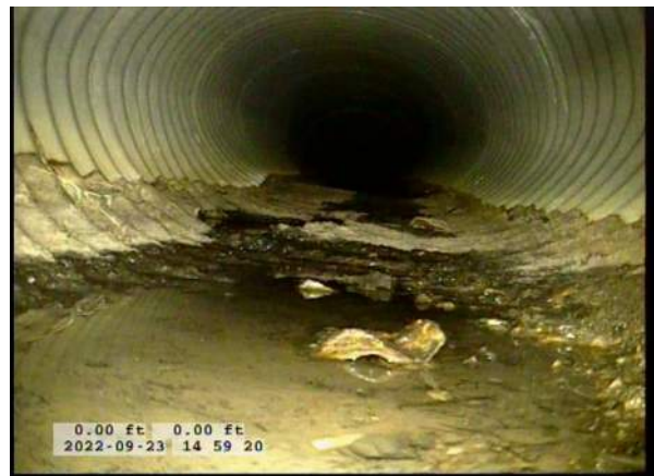
4, 00:00:26, 0.00ft Surface Damage Missing Wall from 5 o'clock to 7 o'clock, within 8 inch, Start / BOTTOM OF PIPE HAS BEGUN TO RUST AWAY
