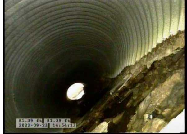
10, 00:05:13, 81.39ft Miscellaneous Survey Abandoned / BOTTOM OF PIPE MISSING, OVERLAPPED WITH RUN FROM OPPOSITE DIRECTION
