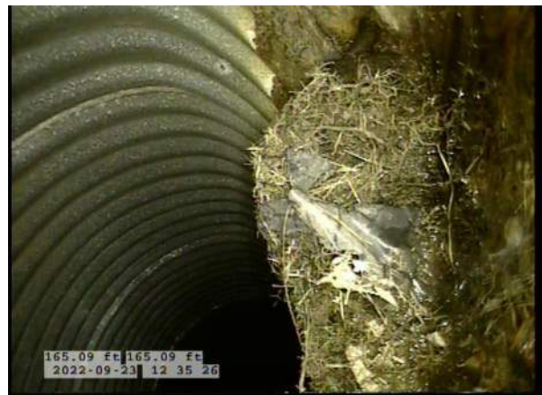
16, 00:13:57, 165.09ft Roots Medium Joint from 4 o'clock to 8 o'clock, 15% of cross sectional area, within 8 inch
