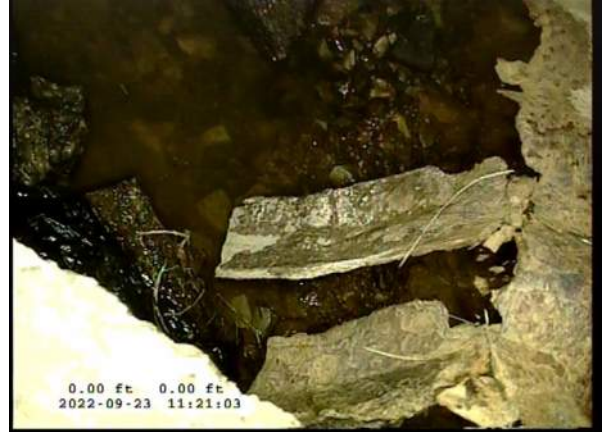
6, 00:01:14, 0.00ft Miscellaneous General Photograph from 5 o'clock to 7 o'clock / BOTTOM OF PIPE MISSING
