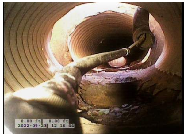
4, 00:00:25, 0.00ft Miscellaneous General Observation / STARTED RUN A COUPLE FEET INTO THE LINE DUE TO BOTTOM OF PIPE MISSING
