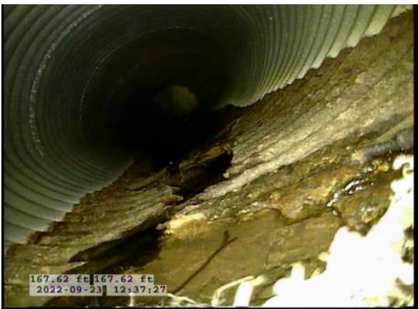
19, 00:15:41, 167.62ft Deposits Attached Encrustation, 5% of cross sectional area from 3 o'clock to 9 o'clock, within 8 inch, Finish / RUST
