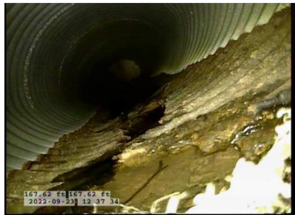
20, 00:15:45, 167.62ft Surface Damage Missing Wall from 5 o'clock to 7 o'clock, within 8 inch, Finish / BOTTOM OF PIPE HAS STARTED TO RUST AWAY
