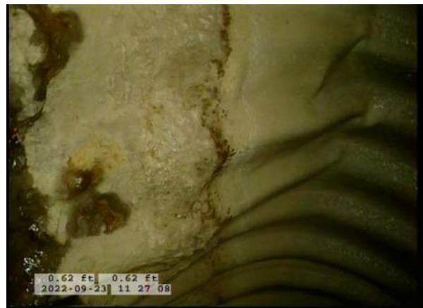
4, 00:00:42, 0.62ft Deformed Flexible Bulging Round, change to: 5% from 7 o'clock to 9 o'clock
