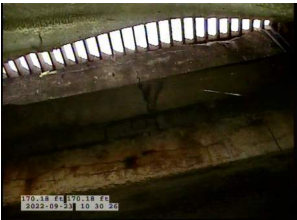
15, 00:08:02, 170.17ft Catch Basin / CB10
