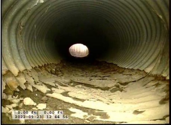
1, 00:00:10, 0.00ft Catch Basin / CB5
