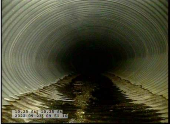
5, 00:00:44, 10.25ft Deposits Attached Encrustation, 5% of cross sectional area from 5 o'clock to 7 o'clock, within 8 inch, Start / RUST
