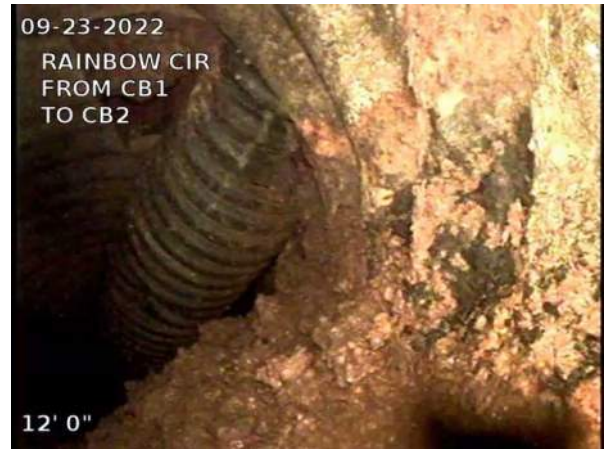
10, 00:01:24, 12.00ft Obstruction External Pipe or Cable, 40% of cross sectional area from 12 o'clock to 12 o'clock / 10 INCH CPP FROM CB2
