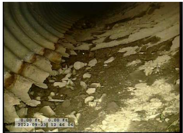
4, 00:00:31, 0.00ft Surface Damage Missing Wall from 5 o'clock to 7 o'clock, within 8 inch, Start / BOTTOM OF PIPE HAS BEGUN RUSTING AWAY
