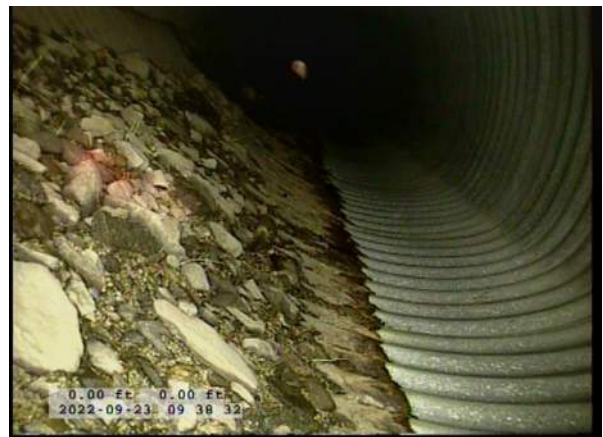
4, 00:00:34, 0.00ft Deposits Attached Encrustation, 5% of cross sectional area from 5 o'clock to 7 o'clock, within 8 inch, Start / RUST
