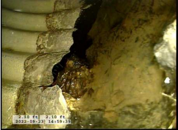
5, 00:00:26, 0.00ft Surface Damage Missing Wall from 5 o'clock to 7 o'clock, within 8 inch, Start / BOTTOM OF PIPE HAS BEGUN TO RUST AWAY
