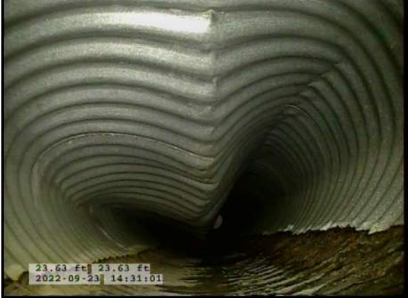
9, 00:01:57, 23.63ft Miscellaneous Survey Abandoned / COLLAPSED PIPE, OVERLAPPED WITH RUN FROM OPPOSITE DIRECTION
