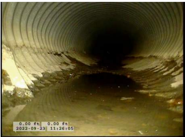
3, 00:00:24, 0.00ft Deposits Attached Encrustation, 5% of cross sectional area from 4 o'clock to 8 o'clock, within 8 inch, Start / RUST
