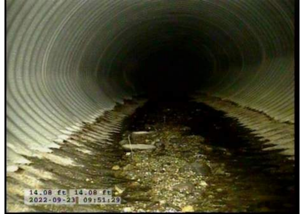
6, 00:00:59, 14.08ft Deposits Settled Compacted, 5% of cross sectional area at 6 o'clock, within 8 inch, Start
