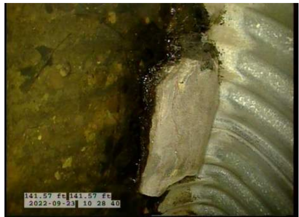
12, 00:06:37, 141.57ft Obstruction Rocks, 5% of cross sectional area at 7 o'clock
