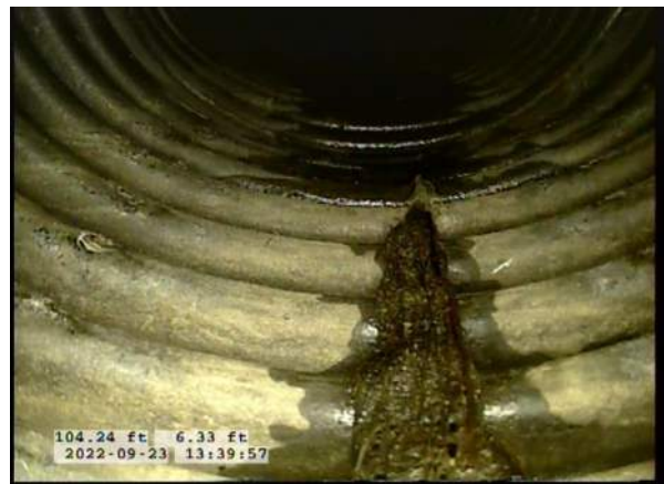
8, 00:01:29, 6.33ft Roots Fine Joint at 6 o'clock, within 8 inch
