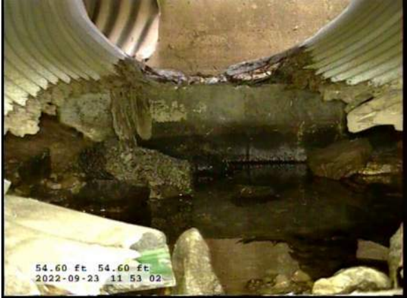
17, 00:07:23, 54.60ft Surface Damage Missing Wall from 5 o'clock to 7 o'clock / BOTTOM OF PIPE MISSING JUST BEFORE CB7
