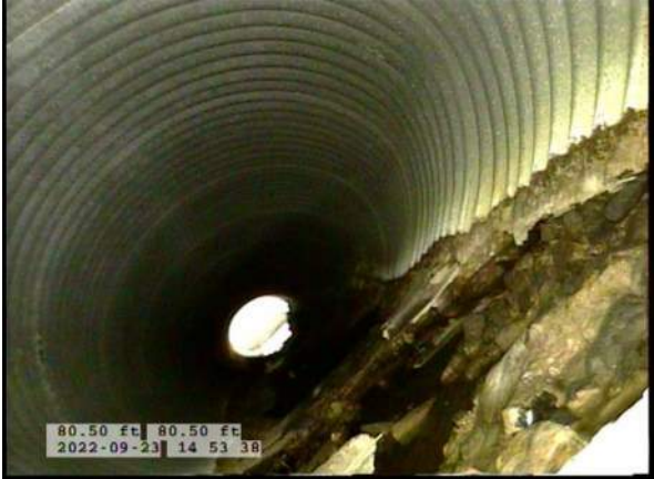
9, 00:05:10, 80.50ft Surface Damage Missing Wall from 5 o'clock to 7 o'clock, within 8 inch, Finish / BOTTOM OF PIPE HAS BEGUN TO RUST AWAY
