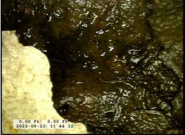
5, 00:00:31, 0.00ft Surface Damage Missing Wall from 5 o'clock to 7 o'clock / BOTTOM OF PIPE HAS RUSTED AWAY AT START OF LINE
