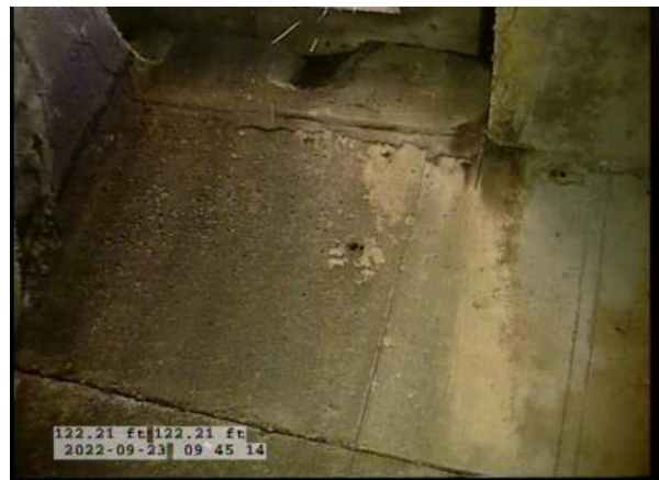
12, 00:06:26, 122.21ft Deposits Attached Encrustation, 5% of cross sectional area from 5 o'clock to 7 o'clock, within 8 inch, Finish / RUST
