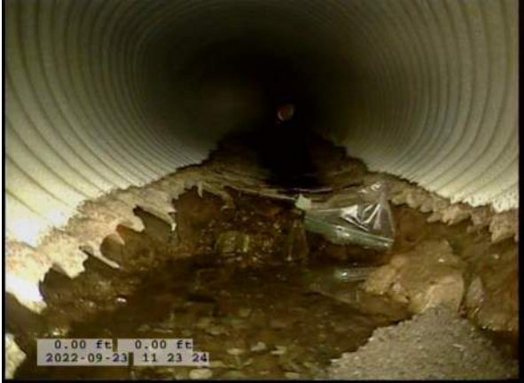
9, 00:02:30, 0.00ft Miscellaneous Survey Abandoned / BOTTOM OF PIPE MISSING, CRAWLER CANNOT ENTER LINE
