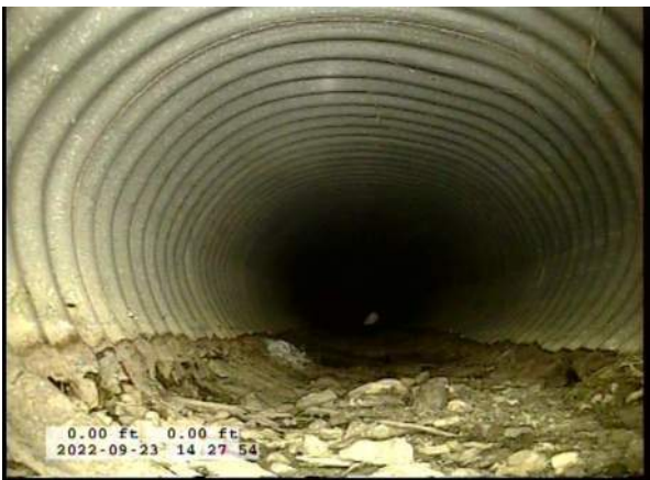
3, 00:00:17, 0.00ft Deposits Attached Encrustation, 5% of cross sectional area from 5 o'clock to 7 o'clock, within 8 inch, Start / RUST
