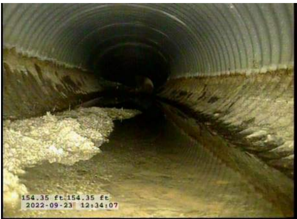
15, 00:12:53, 154.35ft Deposits Settled Fine, 5% of cross sectional area from 6 o'clock to 7 o'clock, within 8 inch, Start
