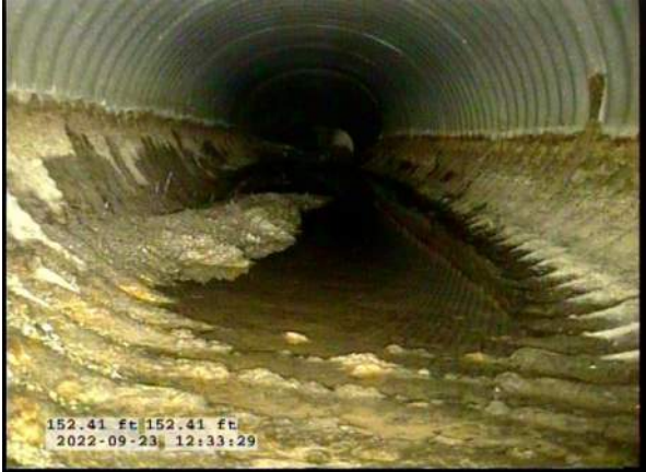
13, 00:12:38, 152.41ft Deposits Attached Encrustation, 5% of cross sectional area from 5 o'clock to 7 o'clock, within 8 inch, Finish / RUST
