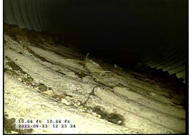
10, 00:02:44, 10.64ft Surface Damage Missing Wall from 5 o'clock to 7 o'clock, within 8 inch, Start / BOTTOM OF PIPE HAS STARTED TO RUST AWAY
