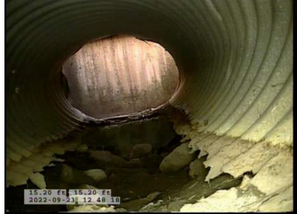
6, 00:01:56, 15.20ft Miscellaneous General Photograph from 5 o'clock to 7 o'clock / BOIIOM OF PIPE COMPLETELY MISSING JUST BEFORE CB4
