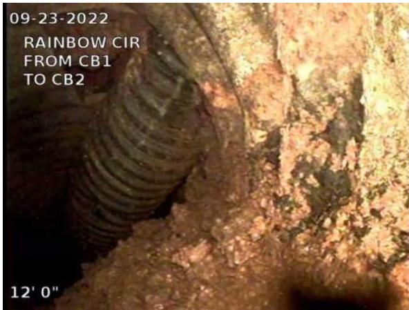
9, 00:00:56, 11.25ft Miscellaneous General Observation / 24 INCH CMP BEING USED AS A CONDUIT FOR THE 10 INCH CPP FROM CB2
