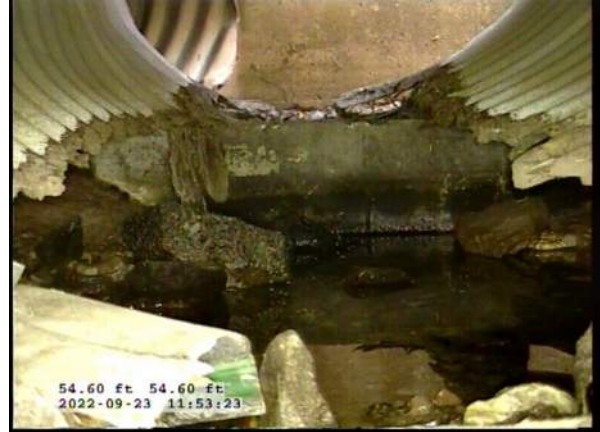
18, 00:07:49, 54.60ft Deposits Attached Encrustation, 5% of cross sectional area from 5 o'clock to 7 o'clock, within 8 inch, Finish / RUST
