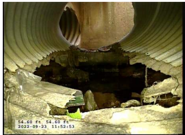
16, 00:07:23, 54.60ft Surface Damage Missing Wall from 5 o'clock to 7 o'clock / BOTTOM OF PIPE MISSING JUST BEFORE CB7
