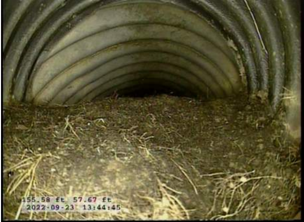
13, 00:05:21, 57.67ft Miscellaneous Survey Abandoned / CANNOT PASS ROOTS
