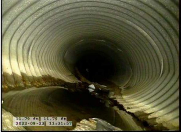
13, 00:03:23, 11.79ft Miscellaneous Survey Abandoned / BOTTOM OF PIPE MISSING, CRAWLER CANNOT PROCEED
