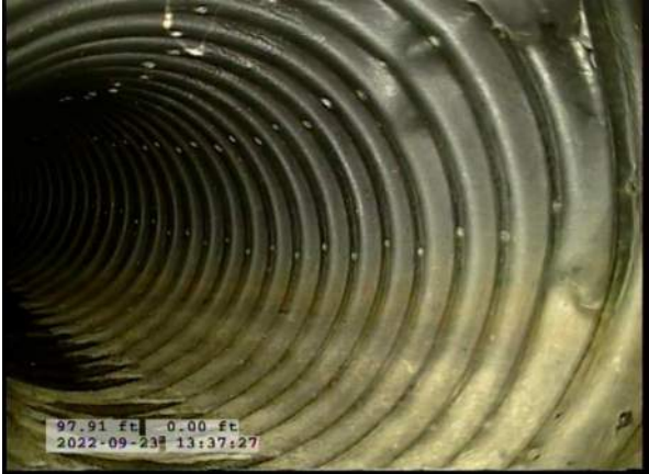
1, 00:00:10, 0.00ft Catch Basin / CB2
