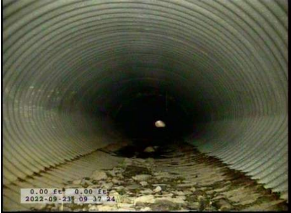
1, 00:00:09, 0.00ft Catch Basin / CB11
