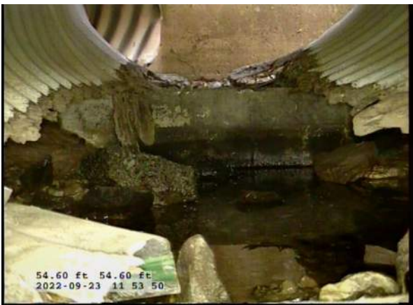
19, 00:07:52, 54.60ft Miscellaneous Survey Abandoned / BOTTOM OF PIPE MISSING, CRSAWLER CANNOT PROCEED
