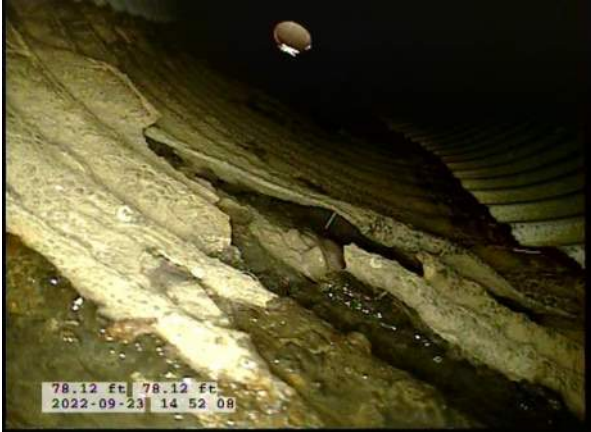
5, 00:00:29, 0.00ft Surface Damage Missing Wall from 5 o'clock to 7 o'clock, within 8 inch, Start / BOTTOM OF PIPE HAS BEGUN TO RUST AWAY
