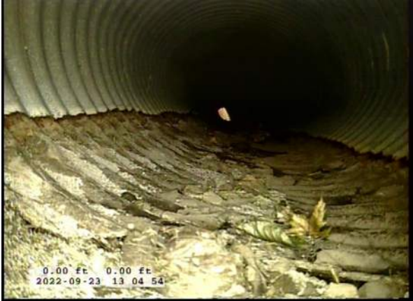
5, 00:00:37, 0.00ft Surface Damage Missing Wall from 5 o'clock to 7 o'clock, within 8 inch, Start / BOTTOM OF PIPE HAS BEGUN RUSTING AWAY
