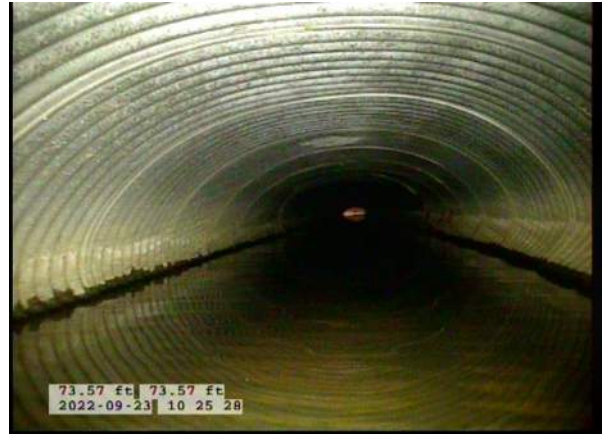
10, 00:04:25, 73.57ft Deposits Settled Compacted, 10% of cross sectional area from 5 o'clock to 7 o'clock, within 8 inch, Finish
