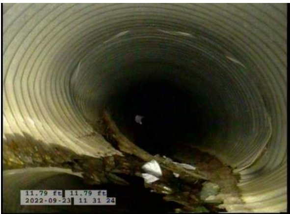
11, 00:03:20, 11.79ft Deposits Attached Encrustation, 5% of cross sectional area from 4 o'clock to 8 o'clock, within 8 inch, Finish / RUST
