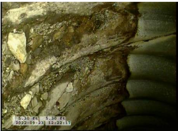
7, 00:02:12, 5.30ft Surface Damage Missing Wall from 5 o'clock to 8 o'clock / PIPE HAS STARTED TO RUST AWAY
