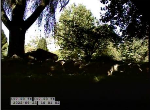
17, 00:07:50, 117.20ft Surface Damage Missing Wall from 5 o'clock to 7 o'clock, within 8 inch, Finish / BOTTOM OF PIPE STARTING TO RUST AWAY, SMALL HOLES FORMING
