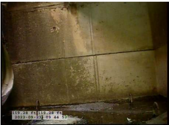
11, 00:06:07, 119.27ft Deposits Settled Gravel, 5% of cross sectional area from 5 o'clock to 7 o'clock, within 8 inch, Finish
