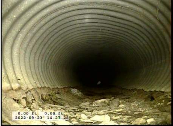
1, 00:00:10, 0.00ft Catch Basin / CB4
