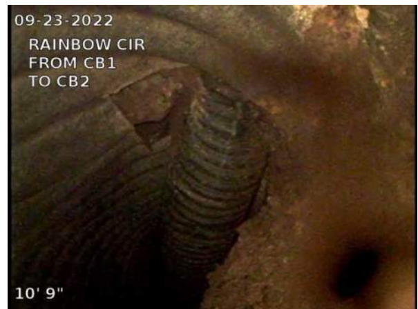
12, 00:01:24, 12.00ft Obstruction Intruding Through Wall, 40% of cross sectional area from 12 o'clock to 12 o'clock / 10 INCH CPP EXITING LINE THROUGH THE WALL OF THE 24 INCH CMP
