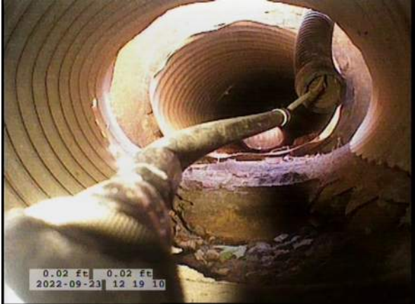
5, 00:00:28, 0.00ft Surface Damage Missing Wall from 5 o'clock to 7 o'clock / CAMERA LOOKING BACKWARDS, BOTTOM OF PIPE MISSING AT START OF LINE
