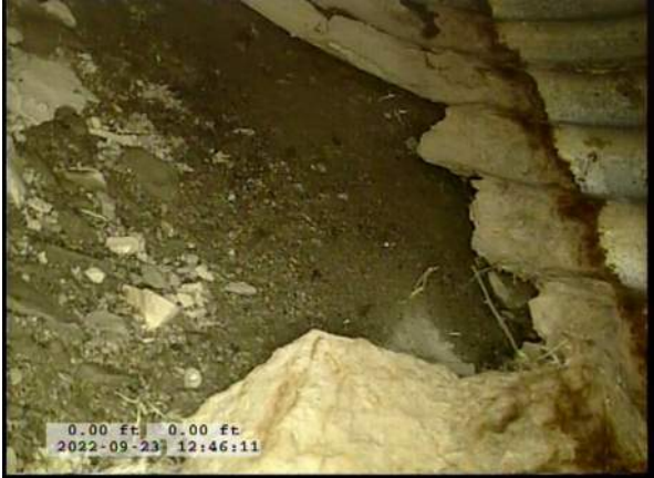
5, 00:00:31, 0.00ft Surface Damage Missing Wall from 5 o'clock to 7 o'clock, within 8 inch, Start / BOTTOM OF PIPE HAS BEGUN RUSTING AWAY
