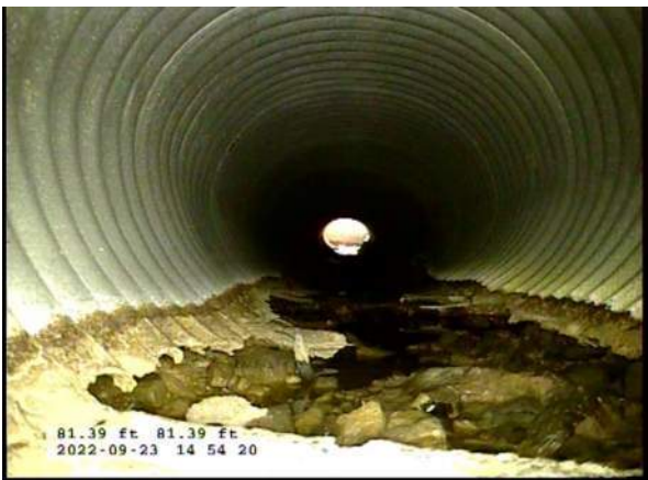
11, 00:05:13, 81.39ft Miscellaneous Survey Abandoned / BOTTOM OF PIPE MISSING, OVERLAPPED WITH RUN FROM OPPOSITE DIRECTION
