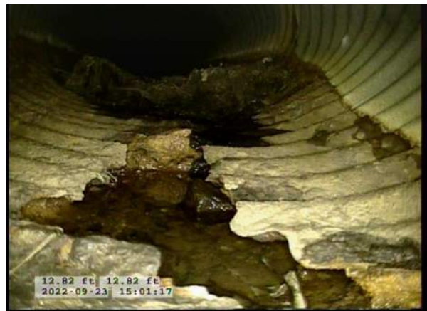
8, 00:01:51, 12.82ft Miscellaneous General Observation / BITTOM OF PIPE COMPLETELY MISSING
