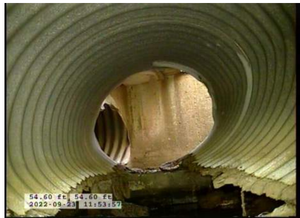
20, 00:07:52, 54.60ft Miscellaneous Survey Abandoned / BOTTOM OF PIPE MISSING, CRSAWLER CANNOT PROCEED
