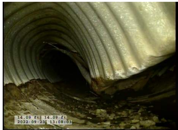
8, 00:03:05, 14.09ft Surface Damage Missing Wall from 5 o'clock to 7 o'clock, within 8 inch, Finish / BOTTOM OF PIPE HAS BEGUN RUSTING AWAY
