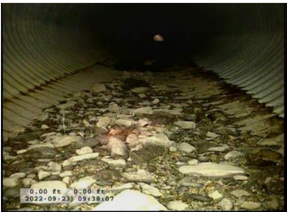
3, 00:00:24, 0.00ft Deposits Settled Gravel, 5% of cross sectional area at 6 o'clock, within 8 inch, Start
