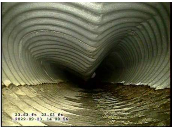
7, 00:01:44, 23.63ft Surface Damage Missing Wall from 5 o'clock to 7 o'clock, within 8 inch, Finish / BOTTOM OF PIPE HAS BEGUN TO RUST AWAY
