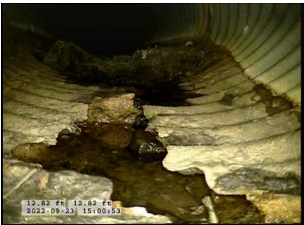
7, 00:01:47, 12.82ft Surface Damage Missing Wall from 5 o'clock to 7 o'clock, within 8 inch, Finish / BOTTOM OF PIPE HAS BEGUN TO RUST AWAY
