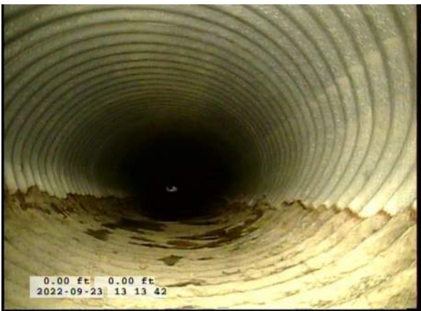
3, 00:00:17, 0.00ft Deposits Attached Encrustation, 5% of cross sectional area from 5 o'clock to 7 o'clock, within 8 inch, Start / RUST
