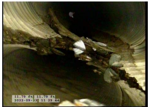
8, 00:02:29, 11.79ft Surface Damage Missing Wall from 5 o'clock to 7 o'clock / BOTTOM OF PIPE HAS RUSTED AWAY
