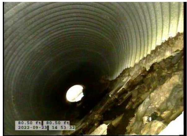
8, 00:05:08, 80.50ft Deposits Attached Encrustation, 5% of cross sectional area from 5 o'clock to 7 o'clock, within 8 inch, Finish / RUST
