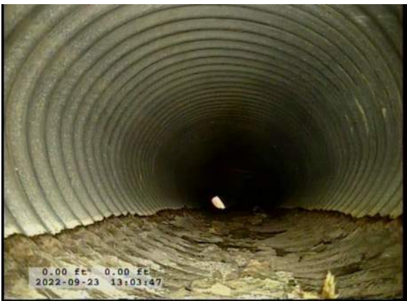
3, 00:00:22, 0.00ft Deposits Attached Encrustation, 5% of cross sectional area from 5 o'clock to 7 o'clock, within 8 inch, Start / RUST
