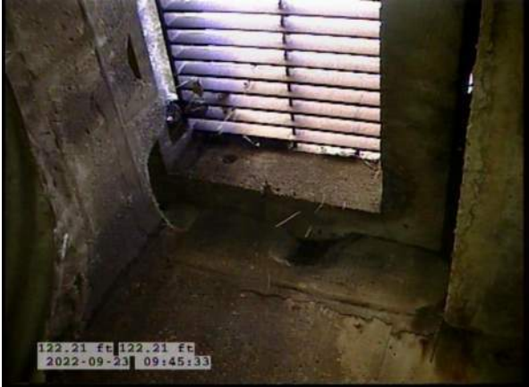
13, 00:06:34, 122.21ft Catch Basin / CB10
