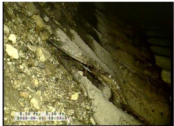
8, 00:02:12, 5.30ft Surface Damage Missing Wall from 5 o'clock to 8 o'clock / PIPE HAS STARTED TO RUST AWAY
