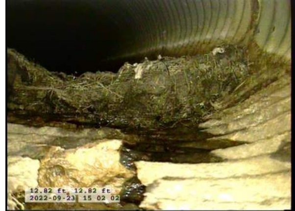
10, 00:02:05, 12.82ft Miscellaneous Survey Abandoned / BOTTOM OF PIPE MISSING, OVERLAPPED WITH RUN FROM OPPOSITE DIRECTION
