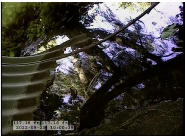
15, 00:07:26, 117.17ft Miscellaneous General Photograph from 5 o'clock to 7 o'clock / BOTTOM OF PIPE COMPLETELY MISSING AT END OF PIPE
