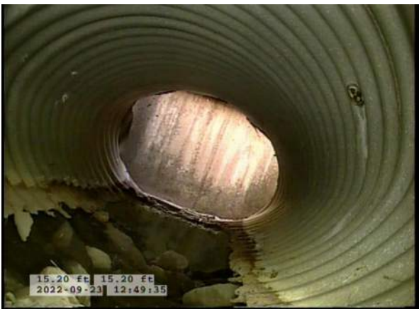
11, 00:02:30, 15.20ft Deposits Attached Encrustation, 5% of cross sectional area from 5 o'clock to 7 o'clock, within 8 inch, Finish / RUST
