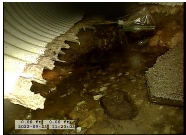
4, 00:00:29, 0.00ft Surface Damage Missing Wall from 5 o'clock to 7 o'clock / BOTTOM OF PIPE HAS RUSTED AWAY
