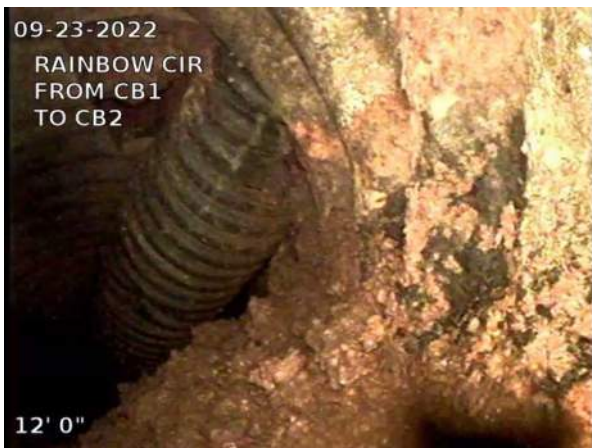
15, 00:01:24, 12.02ft Miscellaneous Survey Abandoned / COULD NOT PUSH CAMERA BEYOND POINT WHERE 10 INCH CPP IS IN THE LINE
