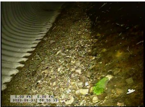
3, 00:00:24, 0.00ft Deposits Settled Compacted, 5% of cross sectional area from 6 o'clock to 7 o'clock, within 8 inch, Start
