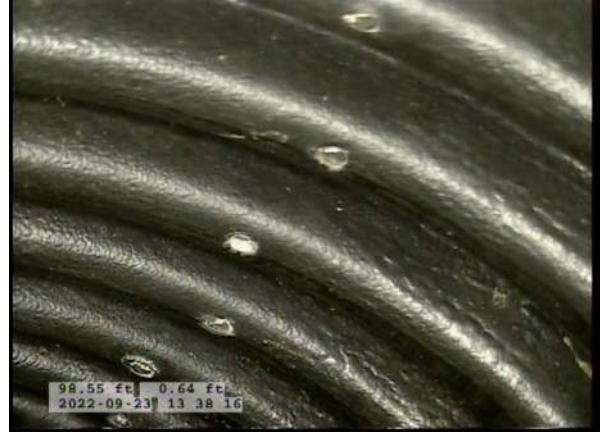
6, 00:00:26, 0.64ft Miscellaneous General Observation / PIPE IS PERFORATED
