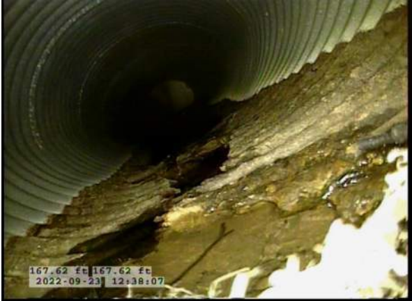
21, 00:15:49, 167.62ft Miscellaneous Survey Abandoned / BOTTOM OF PIPE MISSING, CRAWLER CANNOT PROCEED
