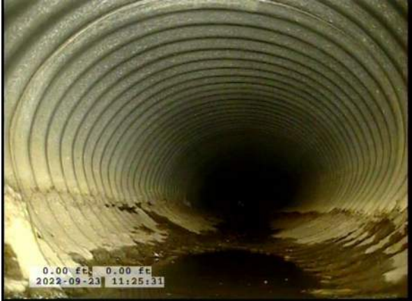
1, 00:00:11, 0.00ft Catch Basin / CB7
