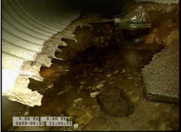
5, 00:01:14, 0.00ft Miscellaneous General Photograph from 5 o'clock to 7 o'clock / BOTTOM OF PIPE MISSING
