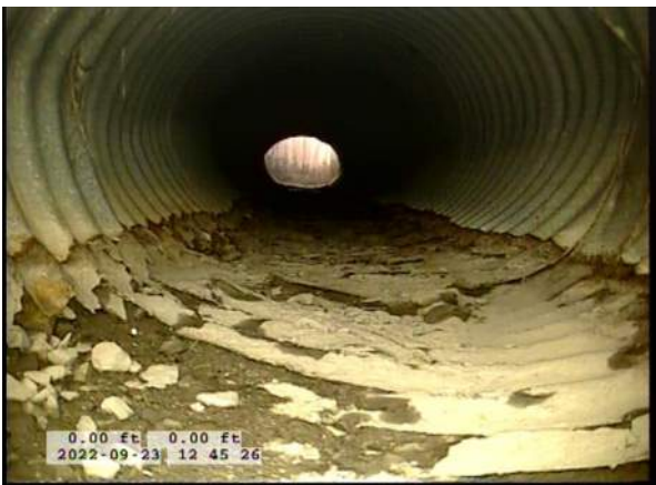
3, 00:00:21, 0.00ft Deposits Attached Encrustation, 5% of cross sectional area from 5 o'clock to 7 o'clock, within 8 inch, Start / RUST
