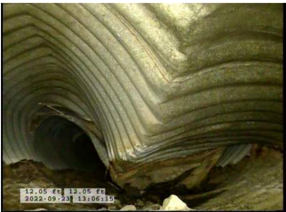
7, 00:01:40, 12.05ft Collapse, 80% of cross sectional area
