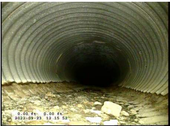
3, 00:00:16, 0.00ft Deposits Attached Encrustation, 5% of cross sectional area from 5 o'clock to 7 o'clock, within 8 inch, Start / RUST
