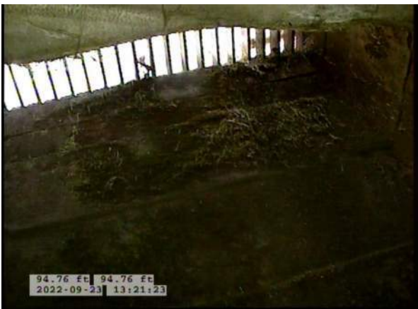
7, 00:07:20, 94.76ft Deposits Attached Encrustation, 5% of cross sectional area from 5 o'clock to 7 o'clock, within 8 inch, Finish / RUST
