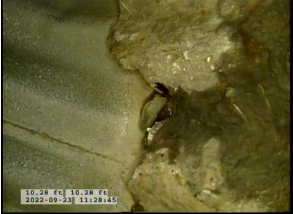
5, 00:01:59, 10.28ft Surface Damage Missing Wall from 7 o'clock to 8 o'clock / SMALL HOLES FORMING
