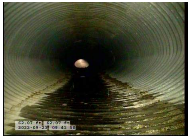
8, 00:03:37, 62.07ft Deposits Settled Gravel, 5% of cross sectional area from 5 o'clock to 7 o'clock, within 8 inch, Finish
