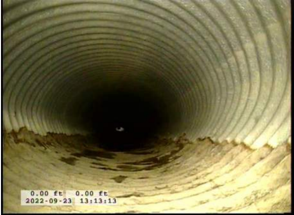
1, 00:00:09, 0.00ft Catch Basin / CB3
