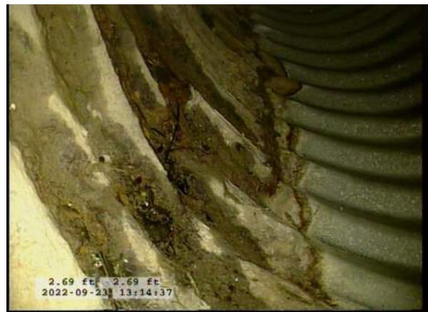
4, 00:00:44, 2.69ft Surface Damage Missing Wall from 5 o'clock to 7 o'clock, within 8 inch, Start / BOTTOM OF PIPE HAS BEGUN RUSTING AWAY
