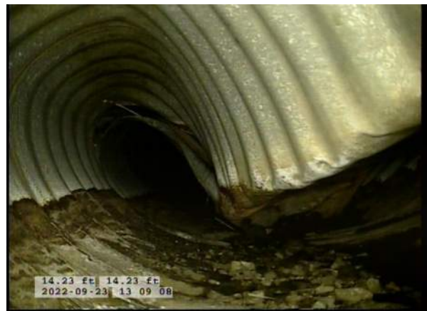
12, 00:03:42, 14.23ft Miscellaneous Survey Abandoned / COLLAPSED PIPE
