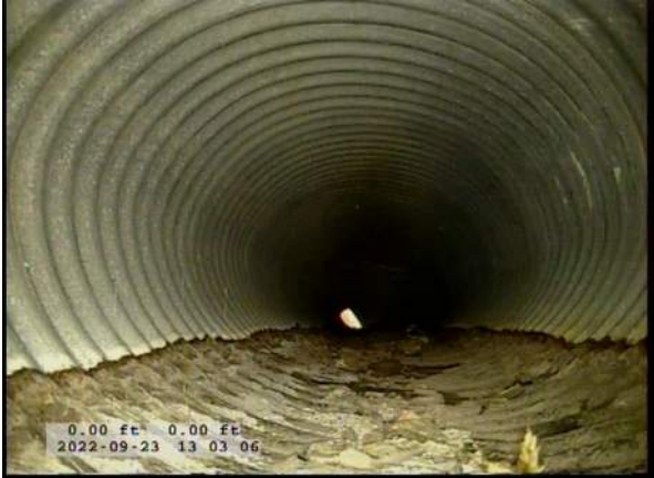
1, 00:00:10, 0.00ft Catch Basin / CB3
