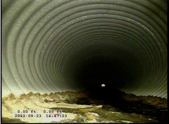
1, 00:00:11, 0.00ft Catch Basin / CB6
