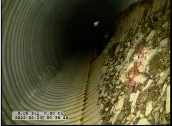
5, 00:00:34, 0.00ft Deposits Attached Encrustation, 5% of cross sectional area from 5 o'clock to 7 o'clock, within 8 inch, Start / RUST
