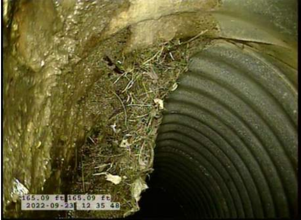
17, 00:13:57, 165.09ft Roots Medium Joint from 4 o'clock to 8 o'clock, 15% of cross sectional area, within 8 inch
