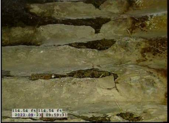
13, 00:06:50, 114.54ft Miscellaneous General Photograph from 5 o'clock to 7 o'clock / BOTTOM OF PIPE RUSTING AWAY
