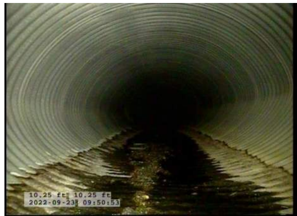
4, 00:00:42, 10.25ft Deposits Settled Compacted, 5% of cross sectional area from 6 o'clock to 7 o'clock, within 8 inch, Finish
