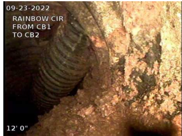
14, 00:01:24, 12.01ft Deposits Attached Encrustation, 5% of cross sectional area from 5 o'clock to 7 o'clock, within 8 inch, Finish / RUST
