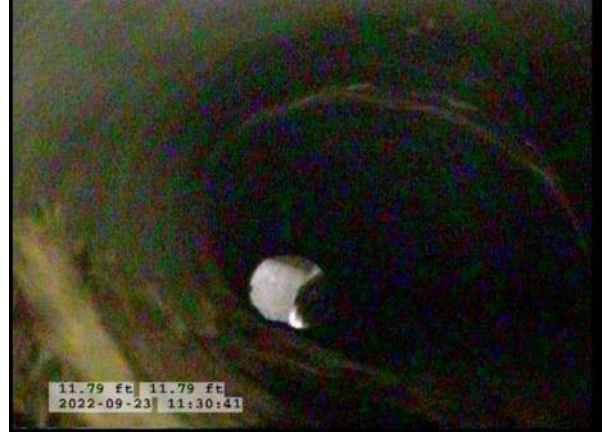
10, 00:02:57, 11.79ft Miscellaneous General Photograph from 12 o'clock to 12 o'clock / ZOOMING CAMERA DOWNPIPE, CB6 VISIBLE
