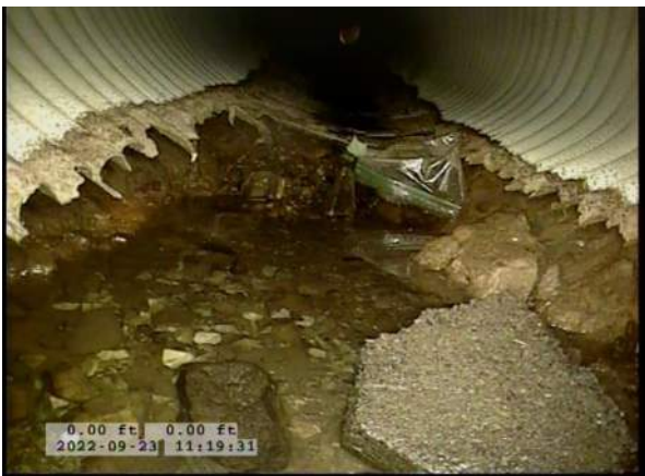
3, 00:00:29, 0.00ft Surface Damage Missing Wall from 5 o'clock to 7 o'clock / BOTTOM OF PIPE HAS RUSTED AWAY
