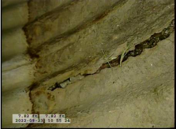
5, 00:01:06, 7.82ft Surface Damage Missing Wall from 5 o'clock to 7 o'clock / BOTTOM OF PIPE STARTING TO RUST AWAY
