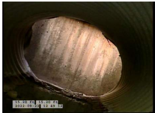
8, 00:02:19, 15.20ft Miscellaneous General Observation / REMAINDER OF LINE AND CB4 VISIBLE
