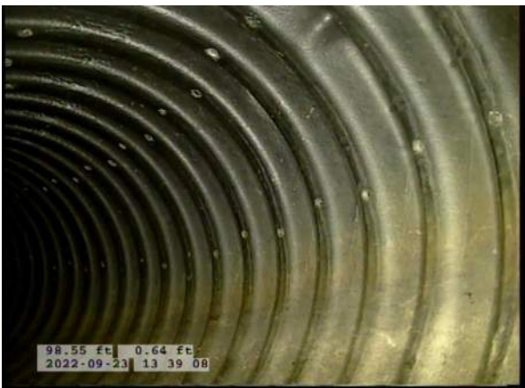
7, 00:00:48, 0.64ft Miscellaneous General Observation / LINE IS BENDING TO THE LEFT
