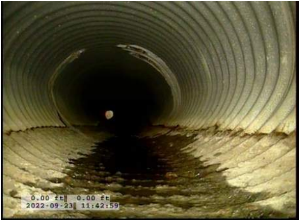
1, 00:00:10, 0.00ft Catch Basin / CB8
