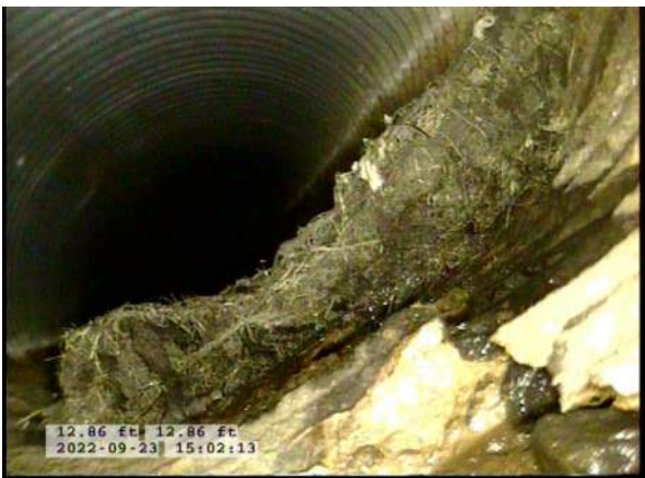
11, 00:02:05, 12.82ft Miscellaneous Survey Abandoned / BOTTOM OF PIPE MISSING, OVERLAPPED WITH RUN FROM OPPOSITE DIRECTION
