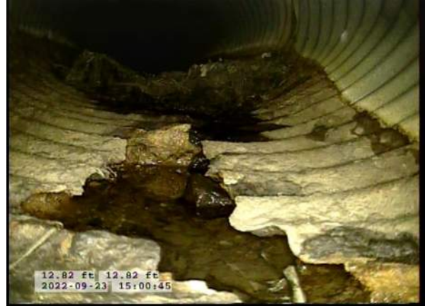
6, 00:01:43, 12.82ft Deposits Attached Encrustation, 5% of cross sectional area from 5 o'clock to 7 o'clock, within 8 inch, Finish / RUST
