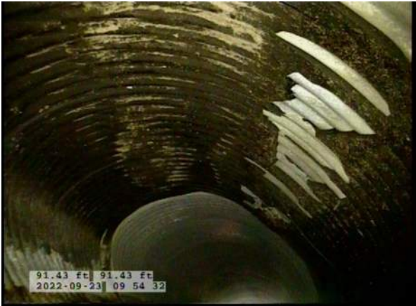
9, 00:03:14, 91.43ft Miscellaneous General Observation / BITUMINOUS COATING ON THIS LENGTH OF THE PIPE
