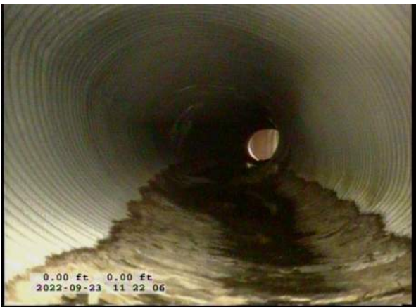
7, 00:01:43, 0.00ft Miscellaneous General Photograph from 12 o'clock to 12 o'clock / ZOOMING CAMERA DOWNPIPE, CB8 VISIBLE
