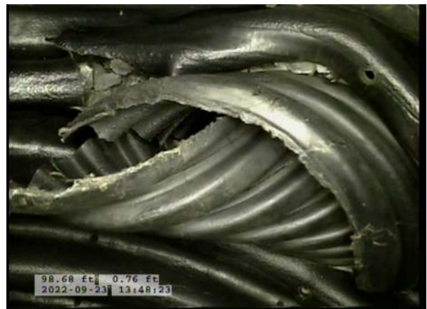
4, 00:05:26, 0.53ft Tap Break-In Defective at 1 o'clock, dia/height: 3inch / CRUSHED END OF PIPE ON LATERAL
