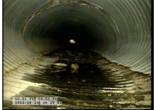
6, 00:01:21, 10.51ft Deposits Settled Gravel, 5% of cross sectional area at 6 o'clock, within 8 inch, Finish
