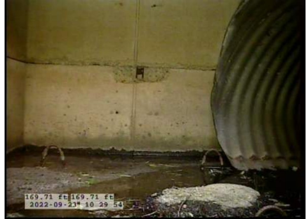
14, 00:07:41, 169.71ft Deposits Attached Encrustation, 5% of cross sectional area from 5 o'clock to 7 o'clock, within 8 inch, Finish / RUST
