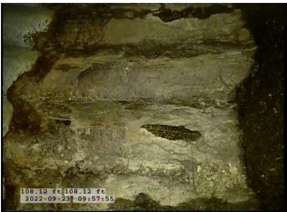
11, 00:05:42, 108.12ft Surface Damage Missing Wall from 5 o'clock to 7 o'clock, within 8 inch, Start / BOTTOM OF PIPE STARTING TO RUST AWAY, SMALL HOLES FORMING
