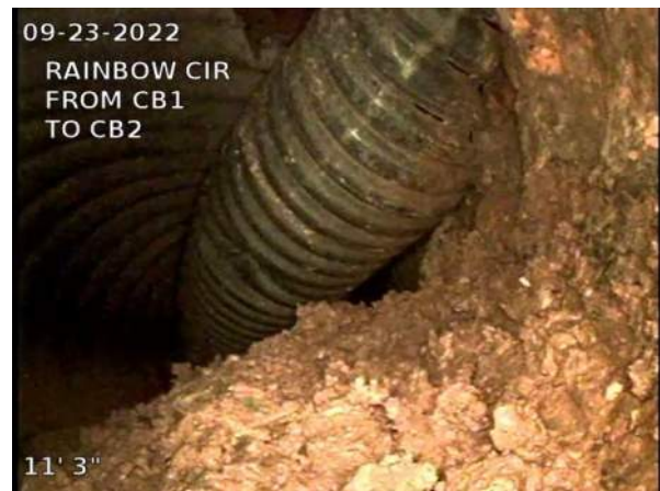
8, 00:00:56, 11.25ft Miscellaneous General Observation / 24 INCH CMP BEING USED AS A CONDUIT FOR THE 10 INCH CPP FROM CB2
