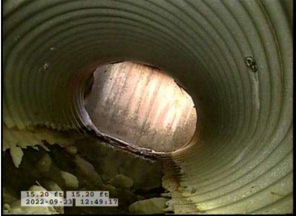
9, 00:02:19, 15.20ft Miscellaneous General Observation / REMAINDER OF LINE AND CB4 VISIBLE
