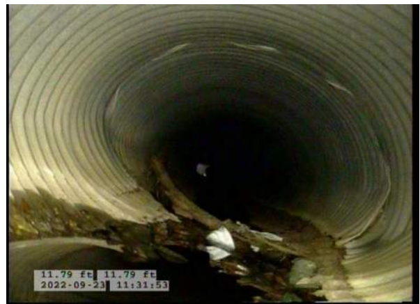
12, 00:03:23, 11.79ft Miscellaneous Survey Abandoned / BOTTOM OF PIPE MISSING, CRAWLER CANNOT PROCEED
