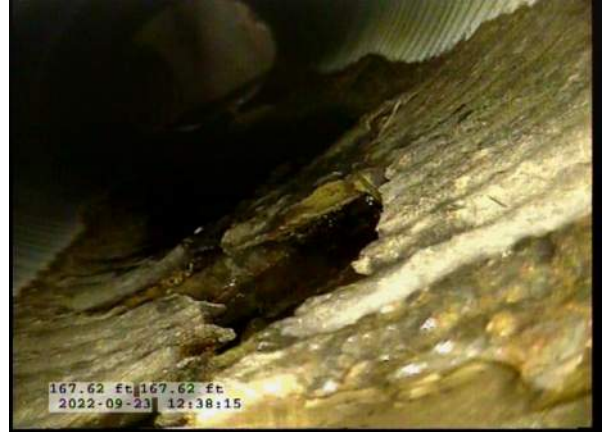
22, 00:15:49, 167.62ft Miscellaneous Survey Abandoned / BOTTOM OF PIPE MISSING, CRAWLER CANNOT PROCEED
