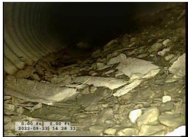
4, 00:00:27, 0.00ft Surface Damage Missing Wall from 5 o'clock to 7 o'clock, within 8 inch, Start / BOTTOM OF PIPE HAS BEGUN TO RUST AWAY
