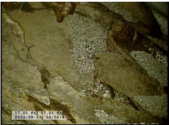
7, 00:01:53, 16.23ft Surface Damage Missing Wall from 5 o'clock to 7 o'clock / BOTTOM OF PIPE RUSTING AWAY
