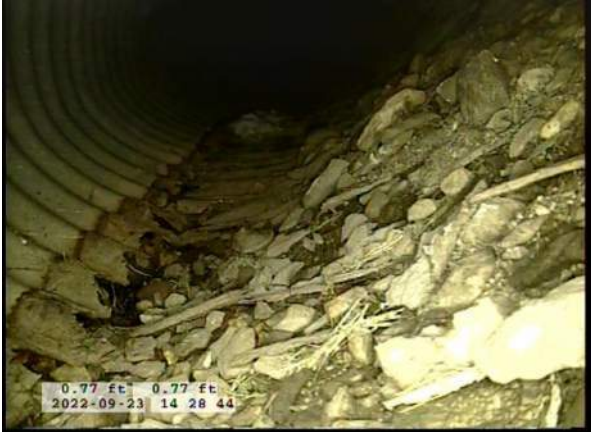
5, 00:00:27, 0.00ft Surface Damage Missing Wall from 5 o'clock to 7 o'clock, within 8 inch, Start / BOTTOM OF PIPE HAS BEGUN TO RUST AWAY
