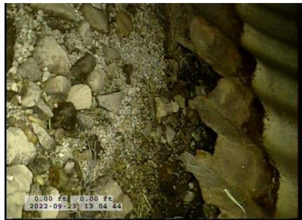
4, 00:00:37, 0.00ft Surface Damage Missing Wall from 5 o'clock to 7 o'clock, within 8 inch, Start / BOTTOM OF PIPE HAS BEGUN RUSTING AWAY
