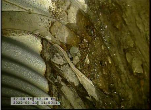
13, 00:05:20, 37.88ft Surface Damage Missing Wall from 4 o'clock to 7 o'clock, within 8 inch, Start / BOTTOM OF PIPE HAS BEGUN RUSTING AWAY
