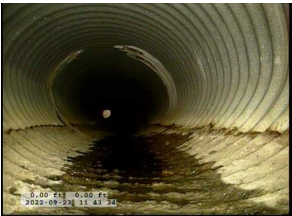
3, 00:00:17, 0.00ft Deposits Attached Encrustation, 5% of cross sectional area from 5 o'clock to 7 o'clock, within 8 inch, Start / RUST
