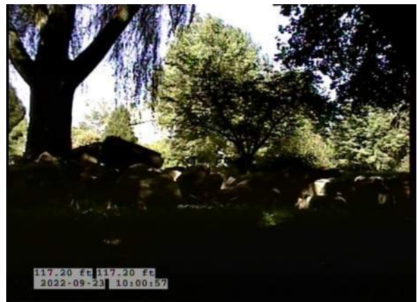
16, 00:07:47, 117.19ft Deposits Attached Encrustation, 5% of cross sectional area from 5 o'clock to 7 o'clock, within 8 inch, Finish / RUST
