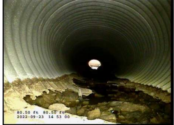
6, 00:04:39, 80.50ft Miscellaneous General Photograph from 5 o'clock to 7 o'clock / BOTTOM OF PIPE COMPLETELY MISSING
