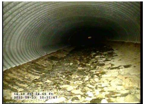
4, 00:01:24, 14.69ft Deposits Settled Gravel, 5% of cross sectional area from 6 o'clock to 7 o'clock, within 8 inch, Start
