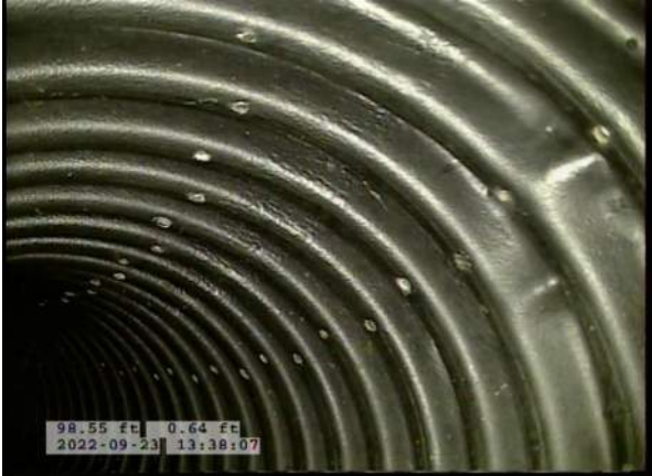
5, 00:00:26, 0.64ft Miscellaneous General Observation / PIPE IS PERFORATED
