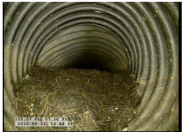
12, 00:04:59, 57.16ft Roots Medium Barrell from 3 o'clock to 9 o'clock, 45% of cross sectional area
