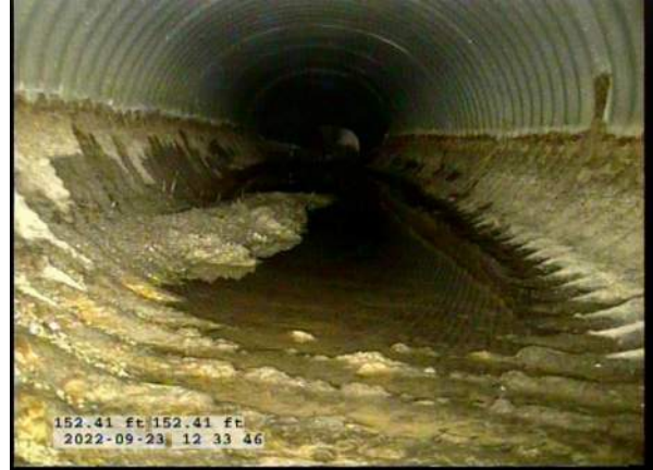
14, 00:12:41, 152.41ft Deposits Attached Encrustation, 5% of cross sectional area from 3 o'clock to 9 o'clock, within 8 inch, Start / RUST
