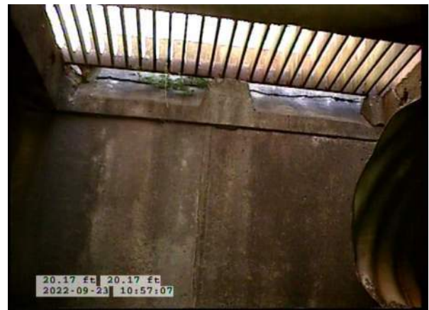
8, 00:02:30, 20.17ft Deposits Attached Encrustation, 5% of cross sectional area from 5 o'clock to 7 o'clock, within 8 inch, Finish
