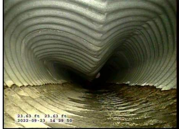
6, 00:01:41, 23.62ft Deposits Attached Encrustation, 5% of cross sectional area from 5 o'clock to 7 o'clock, within 8 inch, Finish / RUST
