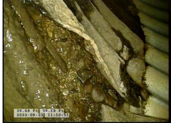
14, 00:05:20, 37.88ft Surface Damage Missing Wall from 4 o'clock to 7 o'clock, within 8 inch, Start / BOTTOM OF PIPE HAS BEGUN RUSTING AWAY
