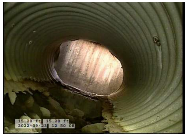
12, 00:02:36, 15.20ft Miscellaneous Survey Abandoned / BOTTOM OF PIPE MISSING, CRAWLER CANNOT PROCEED
