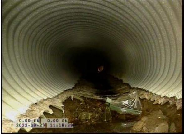
1, 00:00:11, 0.00ft Catch Basin / CB7
