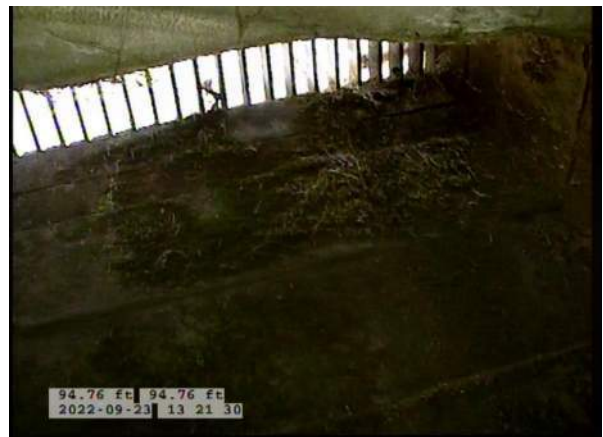
8, 00:07:23, 94.76ft Surface Damage Missing Wall from 5 o'clock to 7 o'clock, within 8 inch, Finish / BOTTOM OF PIPE HAS BEGUN RUSTING AWAY
