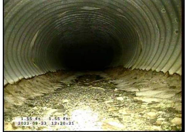
6, 00:00:55, 1.55ft Deposits Settled Compacted, 5% of cross sectional area at 6 o'clock
