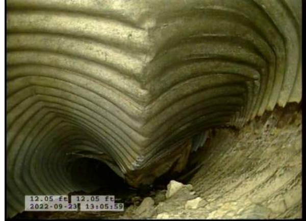
6, 00:01:40, 12.05ft Collapse, 80% of cross sectional area
