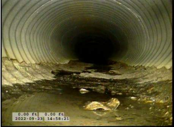
1, 00:00:10, 0.00ft Catch Basin / CB6
