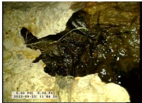
4, 00:00:31, 0.00ft Surface Damage Missing Wall from 5 o'clock to 7 o'clock / BOTTOM OF PIPE HAS RUSTED AWAY AT START OF LINE
