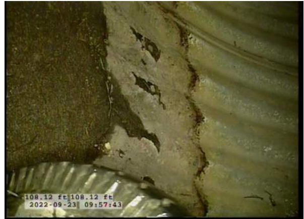
10, 00:05:42, 108.12ft Surface Damage Missing Wall from 5 o'clock to 7 o'clock, within 8 inch, Start / BOTTOM OF PIPE STARTING TO RUST AWAY, SMALL HOLES FORMING
