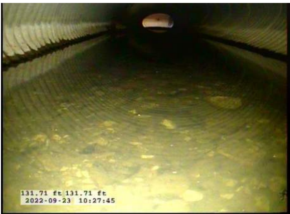
11, 00:06:09, 131.71ft Deposits Settled Compacted, 5% of cross sectional area from 5 o'clock to 7 o'clock, within 8 inch, Start
