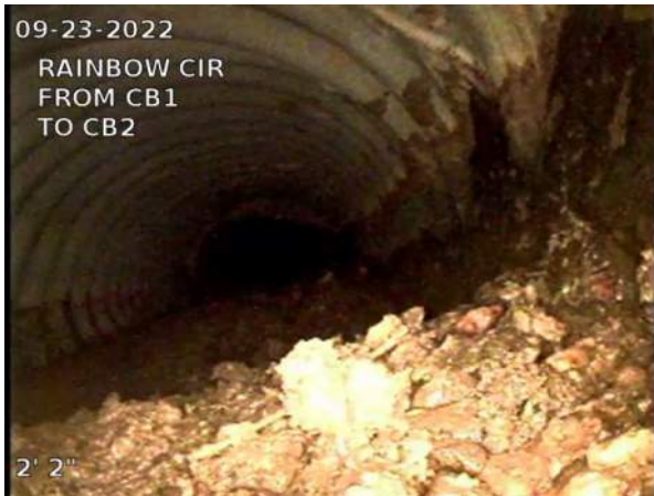
5, 00:00:19, 2.16ft Deposits Settled Gravel, 10% of cross sectional area from 5 o'clock to 7 o'clock, within 8 inch, Start
