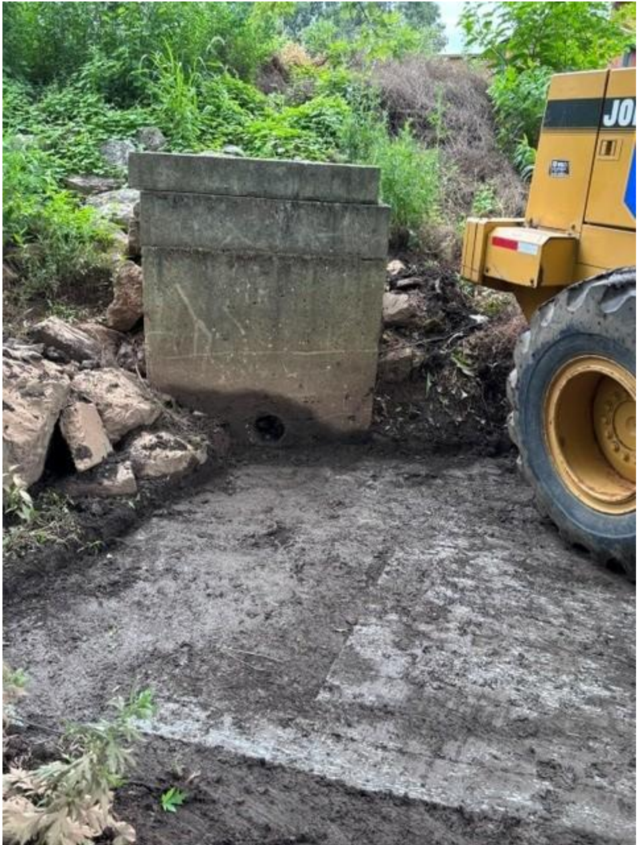
Weldon Rd Storm water before
