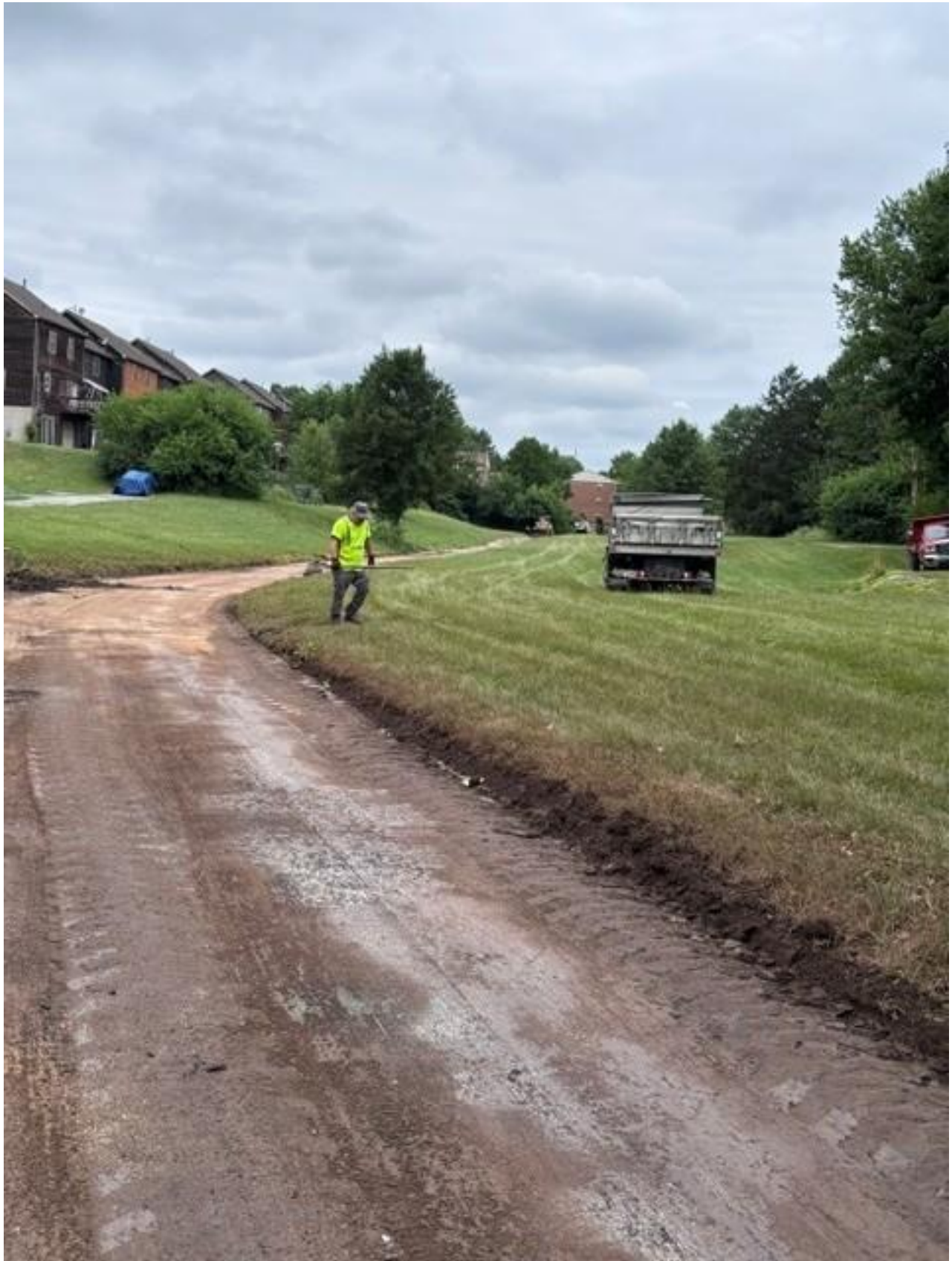
Stanton St Storm damage before
