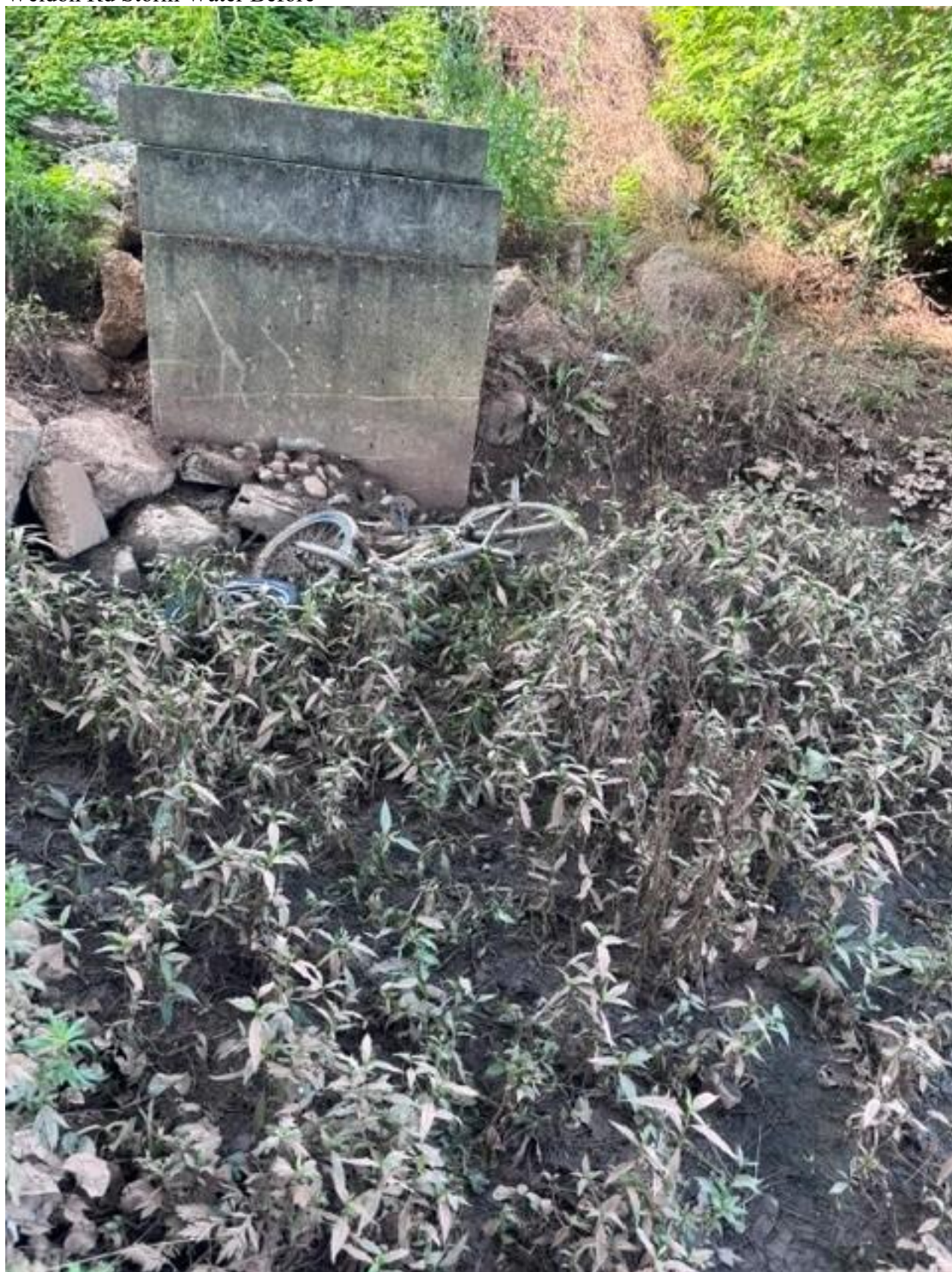
Weldon Rd Storm Water Before
